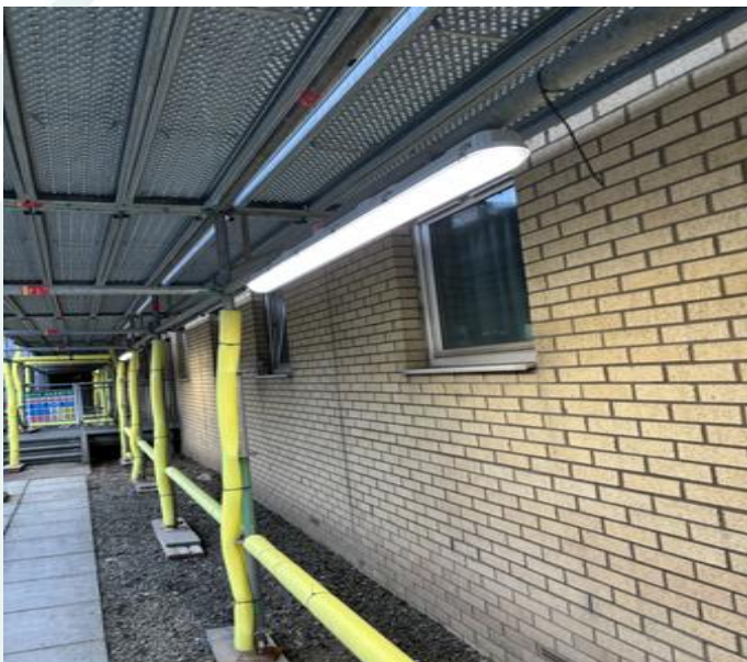
Phase 3 temporary lighting
